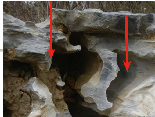
Arrows denote open voids in rock into which soil is being flushed, creating loss of support and surface subsidence.
