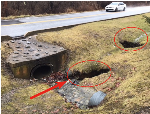
Arrow denotes location where stormwater from culvert is short-circuiting into the ground and has created surface subsidence (red circles).
