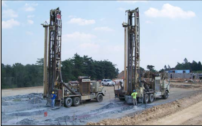
Photograph Above: Eichelbergers Drill Rigs hard at work on the Hotel Hershey job site.
